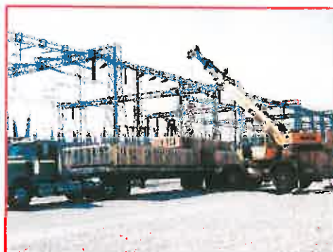
Offloading at the DWP facility. At rough terrain crane easily handles the sensitive parts.
