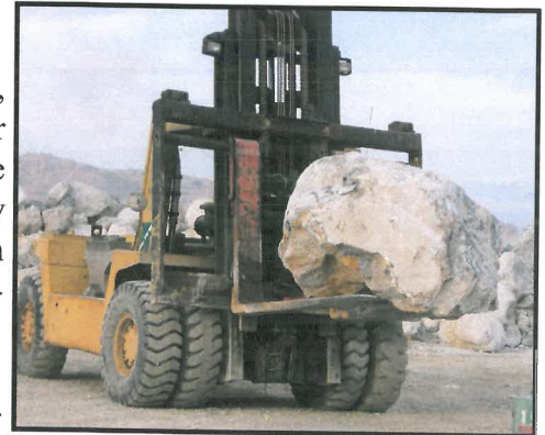
Our 55,000 lb capacity Clark forklift makes handling 7-17 Ton shot rock for breakwater look easy. Note the 13.5 Ton weight of the rock spray painted on it. By pre-weighting these stones, our operator can quickly choose the correct ones needed to yield a maximum legal payload.
