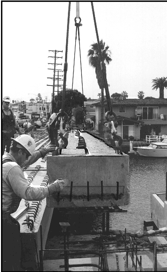
Reinforced-concrete bridge beams being precisely placed over a Newport channel. (Note proximity to residential property and watercrafts.)
