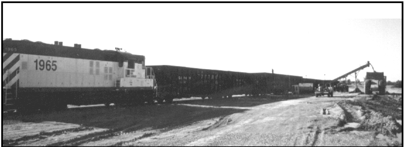
Coast Rail's engine pushes hopper cars across the under rail emptying pit, feeding a conveyor. The sand is loaded into Cat 631 scrapers for hauling to the beach 5 miles away.
